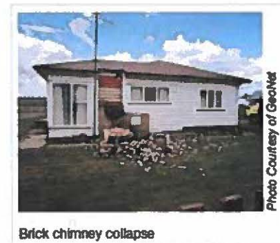
Brick chimney collapse
